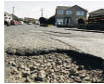
RISK Pothole alert
